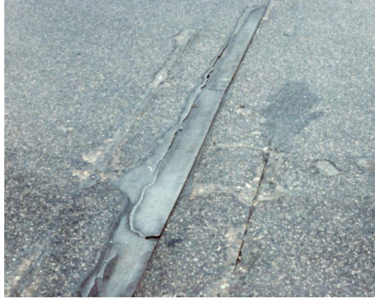
Figure 2.3 Cracked sliding plate joint (Ohio DOT)
