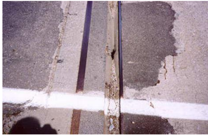
Figure 2.5 Strip seal joint with punctured gland (Baker)
