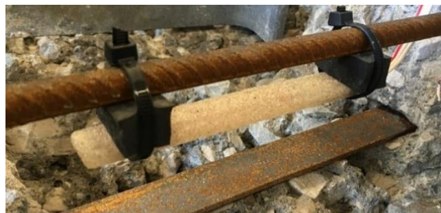
Figure 5.6 Embedded concrete strain gauge (Ruble)
